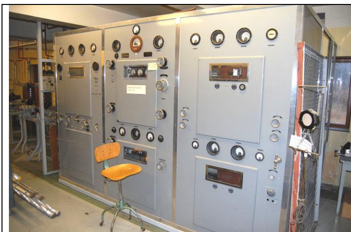
Marconi Transmitter front panel
